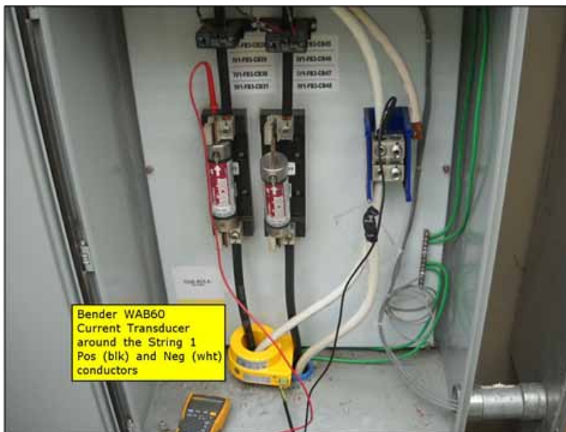
Figure 6. Bender current transducer installed around positive and negative string conductors
